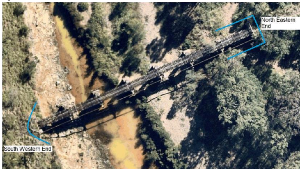
Figure 3.3 View of the Structure ID 1020199 - North Eastern End and South Western End
