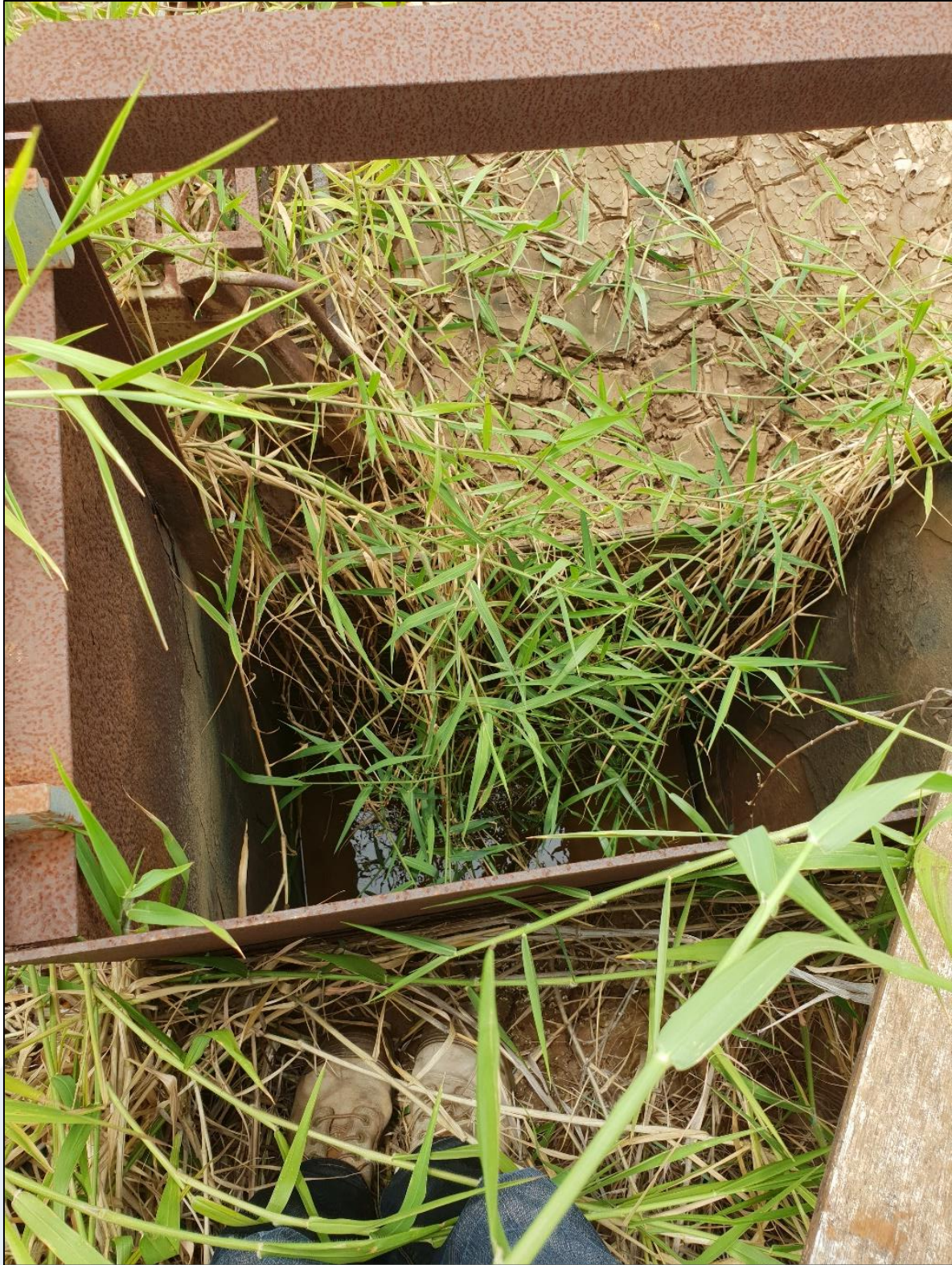
Figure 13. Height-adjustable weir board showing sediment collected upstream (top of photo), and clean water below (middle of photo).
