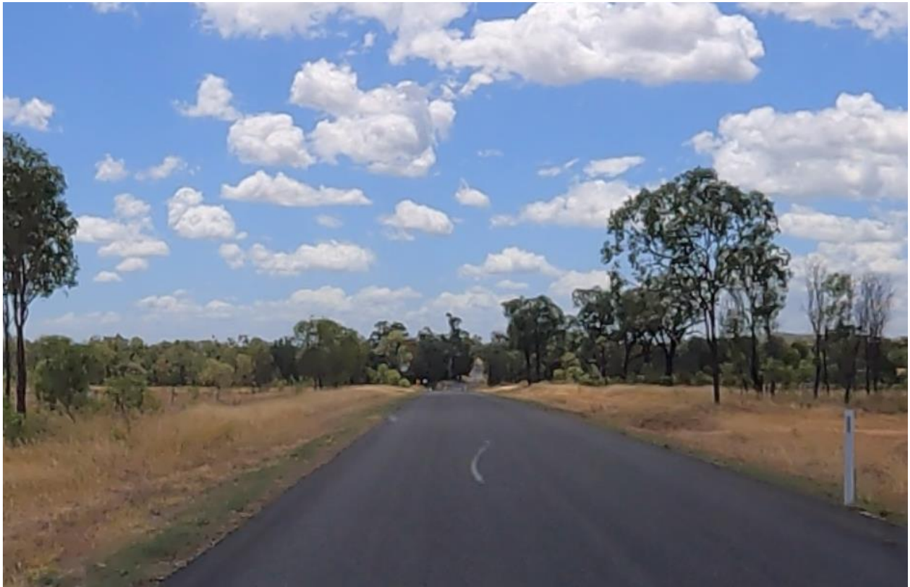
Figure 8-11: Floodway (Ch 5.6km) looking north on approach (400m of sight on approach)
