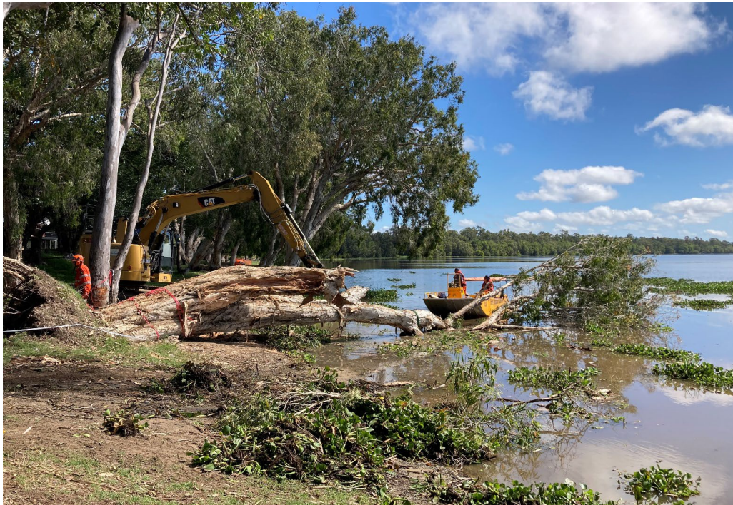
A complex large fallen tree removal at the Ski Gardens was led by the Arboriculture team in collaboration with the SES and Civil Operations. It was a great team effort to all involved.
