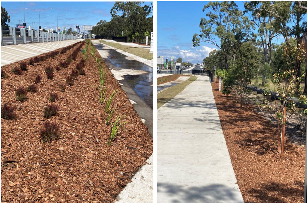
Approximately 2000 plants and 200m 3 of mulching completed by Parks as part of the Farm and Carlton Street (DTMR works). A further 600 plants will be planted in the upcoming weeks.
