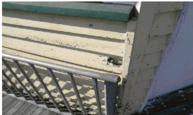
Weather board termite damaged. (Photo 10)
