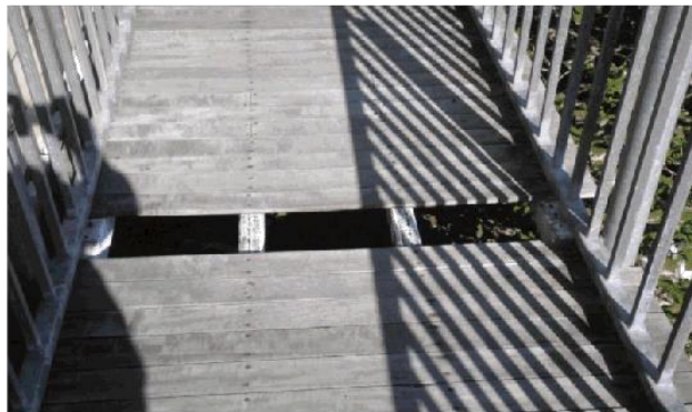
Floor boards missing off the access ramp. (Photo 4)
