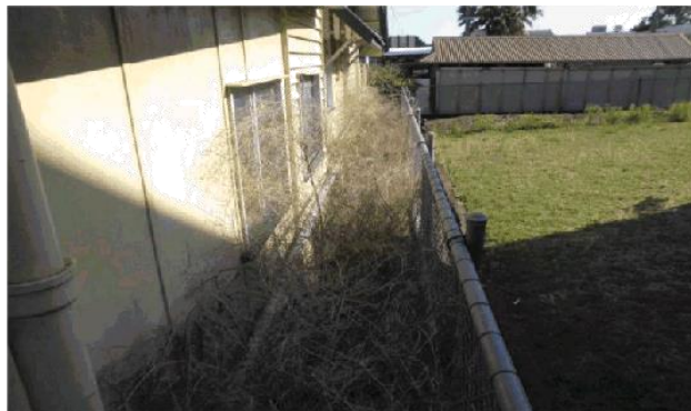
Eastern side of the building overgrown. (Photo 2)
