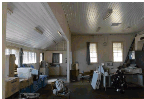
Figure 15: Main office and enclosed former verandah (showing where how the walls have been removed)
