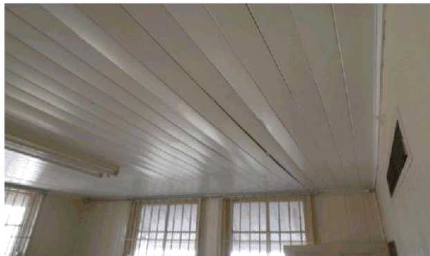
Ceiling boards falling down in office. (Photo 14)
