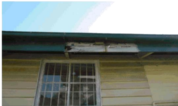
Fascia board rotten. (Photo 8)
