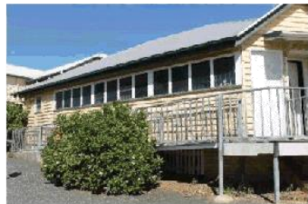
Figure 20: Morgan Street ramp and overgrown plants
