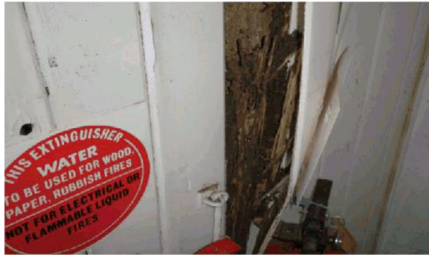
Termite damaged walls. (Photo 13)
