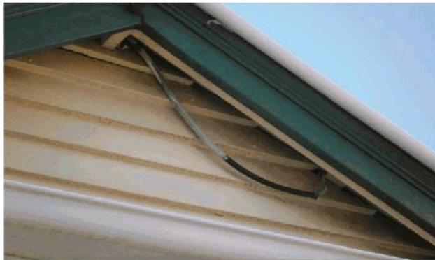
Unsecured electrical cable. (Photo 6)
