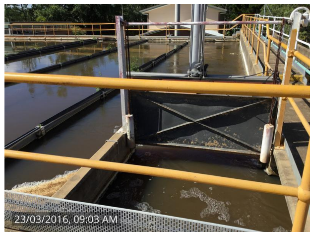
PAC dosing into flocculation tanks
