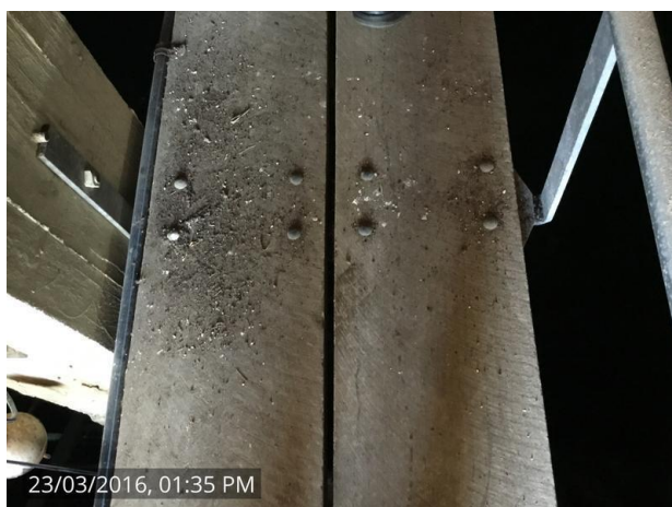
Debris and possible bird faeces inside reservoir
