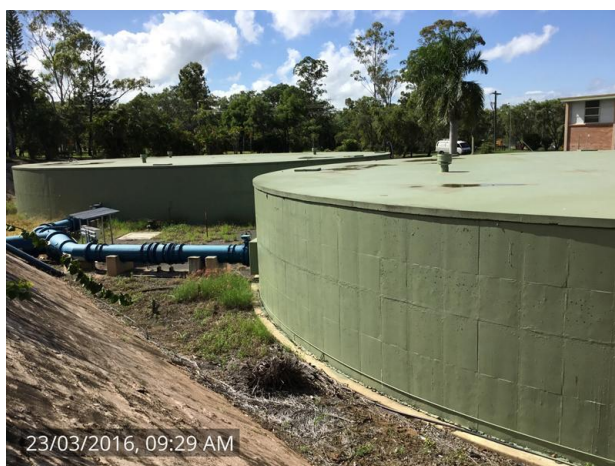
Clear water tanks
