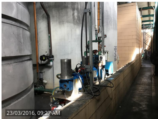
Chemical storage tanks
