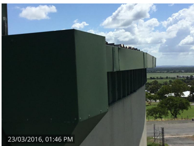
Lifting roofing, may be point of ingress on 20 ML reservoir
