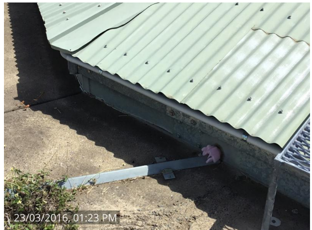
Some lifting of sheeting and hole stuffed with foam
