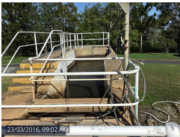
Flume and coagulant dosing
