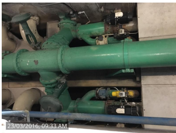
Filter pipework – valves for filter to waste
