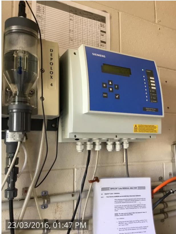
Deplox analyser at Athelstane rechlorination
