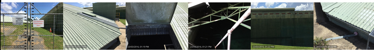
Security gate to Athelstane Reservoirs Inground reservoirs. Hatch fits closely Internal view of ground level reservoir have Terracotta air vents slightly too large holes. Some lifting of roof, hole plugged with foam.
