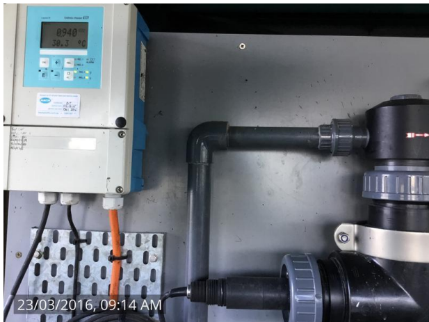
Turbidity meter – tube settlers
