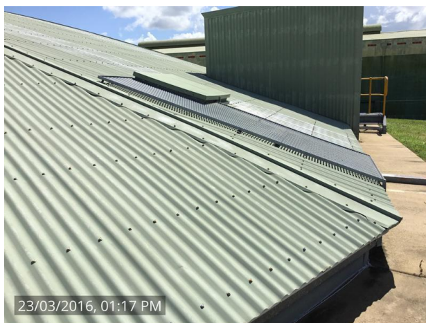
Ground level reservoirs (A and B). Gaps under corrugations
