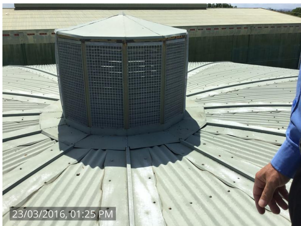
Angle of roof may allow rainwater to run under the whirlybird
