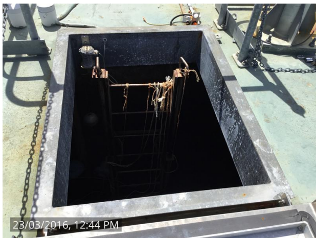
Rogar reservoir – chlorine tablets connected to ropes on ladder
