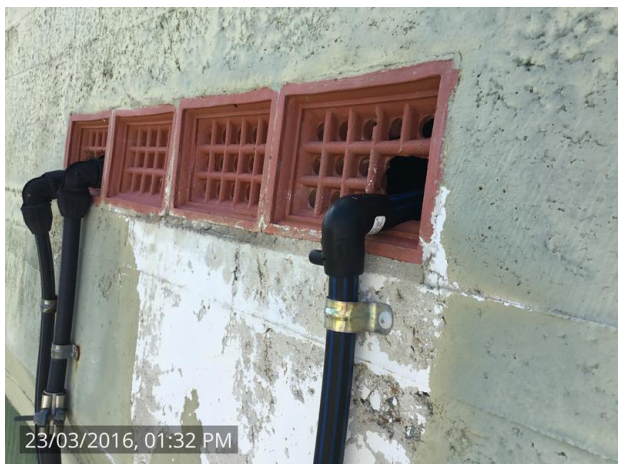
Hole through terracotta is large enough for vermin access
