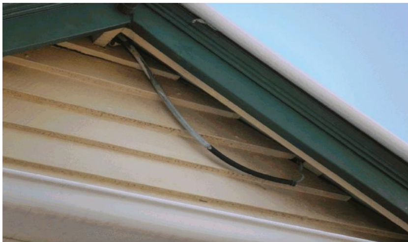
Unsecured electrical cable. (Photo 6)
