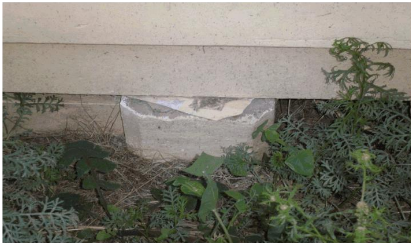
Ant cap not fitted properly will allow termites access. (Photo 16)
