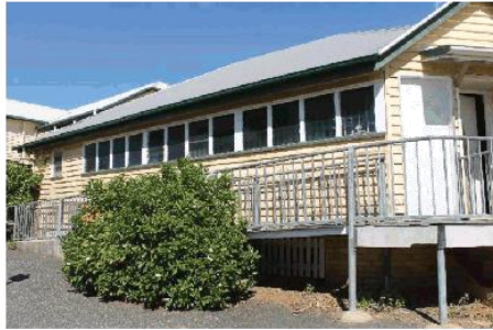
Figure 20: Morgan Street ramp and overgrown plants
