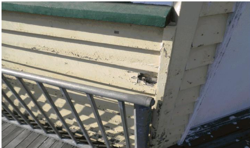
Weather board termite damaged. (Photo 10)
