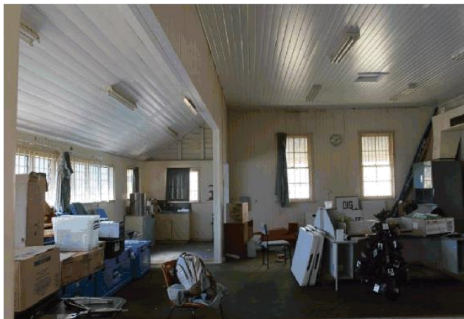
Figure 15: Main office and enclosed former verandah (showing where how the walls have been removed)
