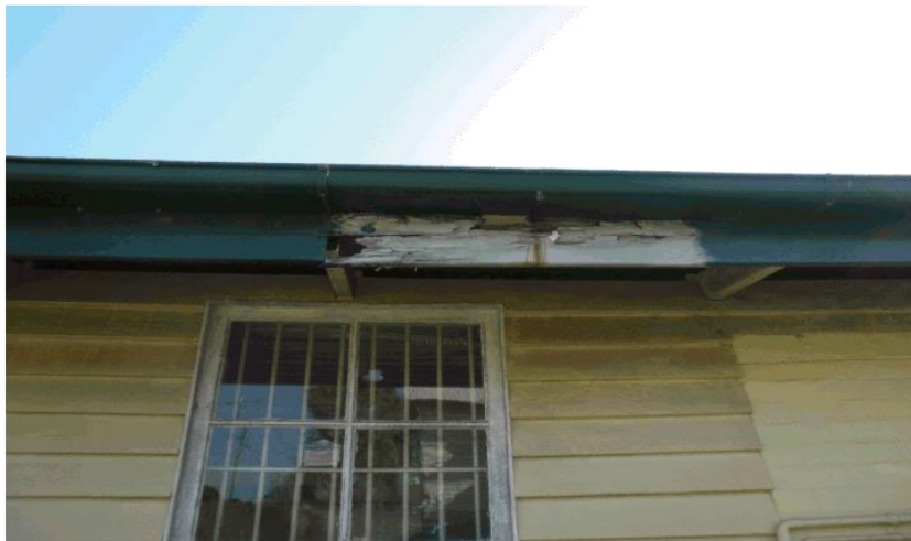
Fascia board rotten. (Photo 8)
