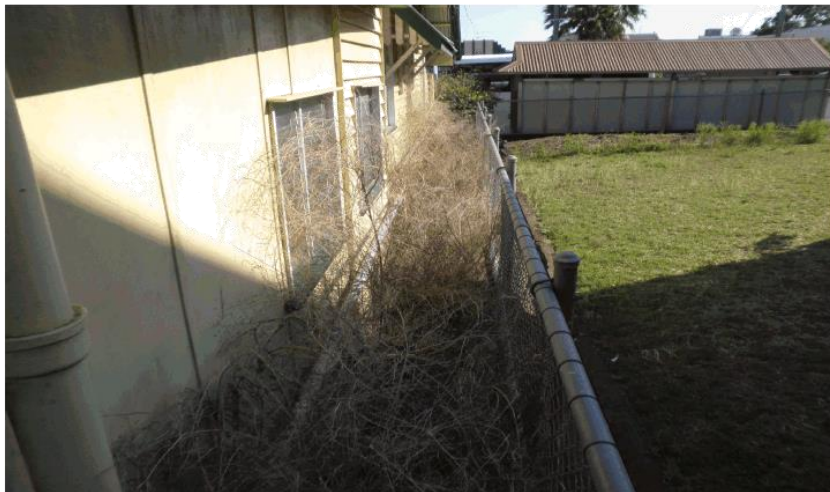
Eastern side of the building overgrown. (Photo 2)
