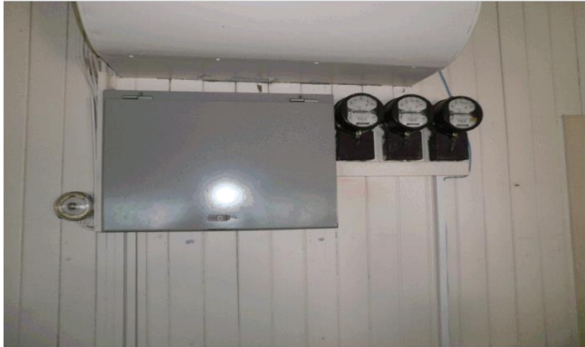
Power board and meters inside the building. (Photo 7)
